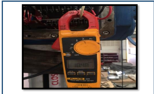
Fig 2. Current of Phase 1 (Before)
