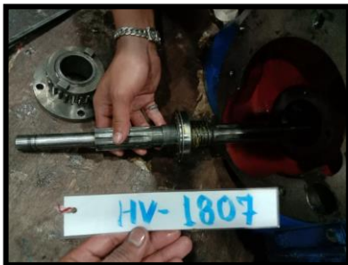
Fig 21. Cleaning Gear Shaft Motor
