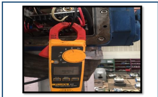
Fig 4. Current of Phase 3 (Before)
