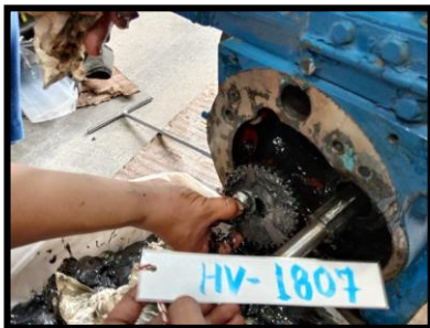
Fig 13. Inspect Gear Shaft Motor
