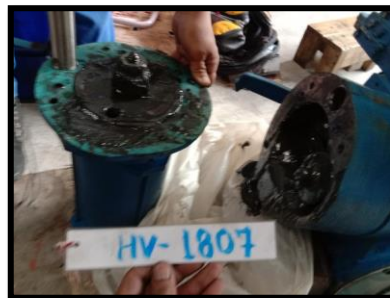
Fig 16. Inspect Motor of the Actuator
