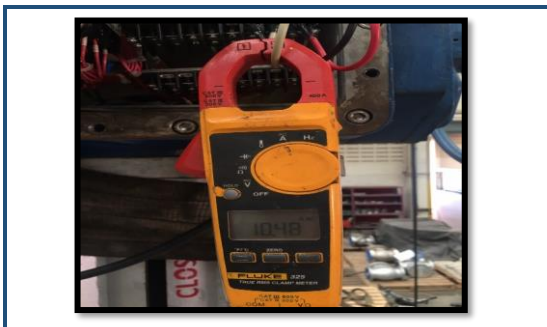
Fig 3. Current of Phase 2 (Before)
