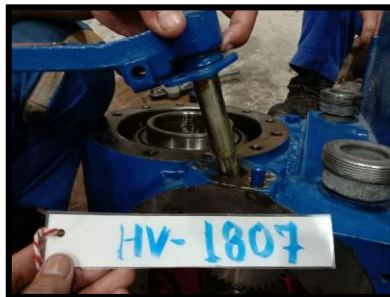
Fig 22. Cleaning Shaft Hand Wheel
